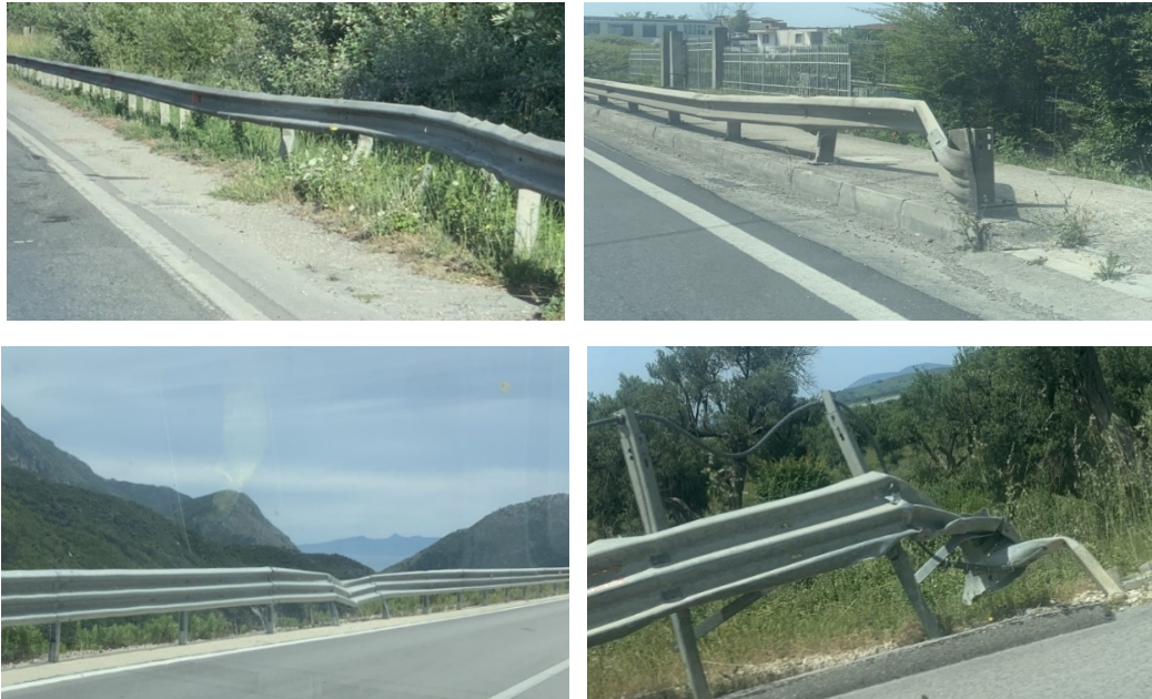
Figure 11. Field inspection of damaged road guardrails.
