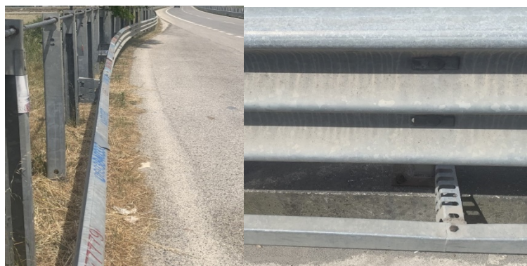
Figure 12. Lack of mounting elements and inaccuracies installation
