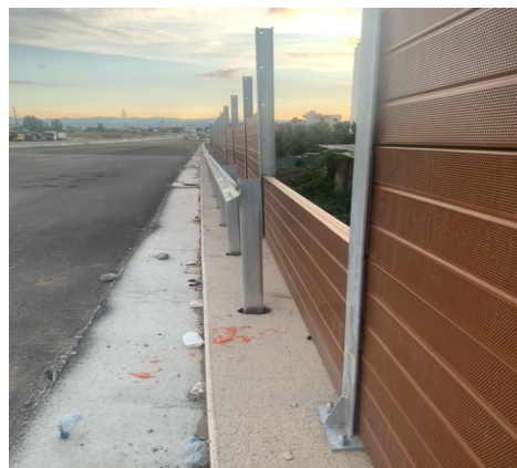
Figure 7. Acoustic panel mounted on safety guardrails.
