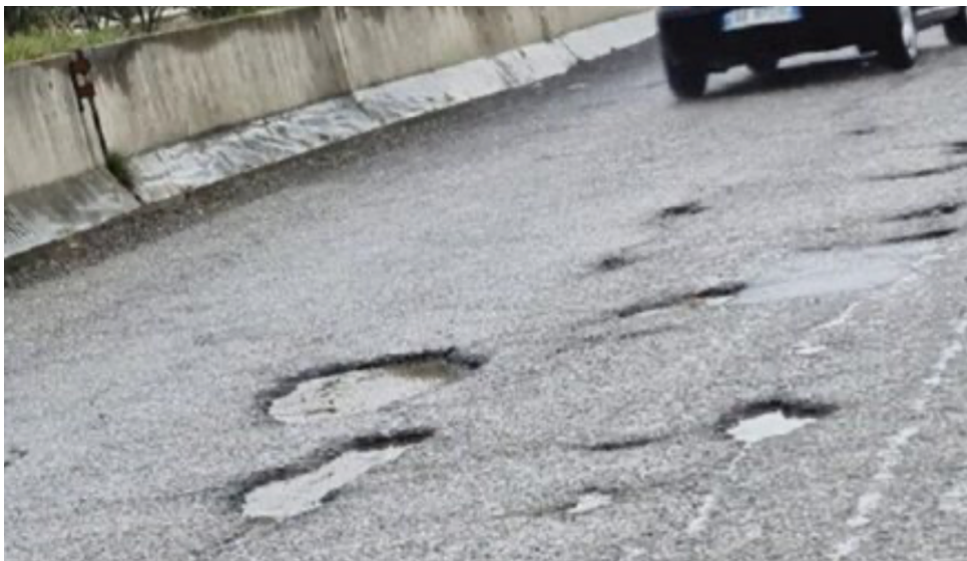
Figure 3. Illustrative photo of road surface defects, highway Tirana-Durres in Albania
