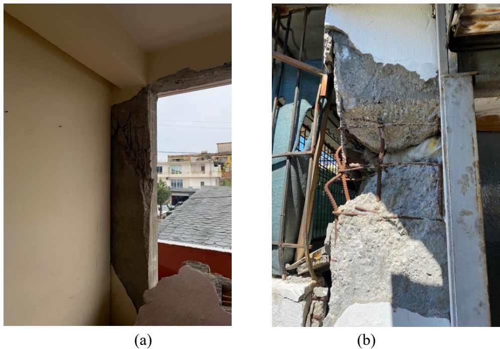
Figure 2. The damaged columns of concrete structures (a) internal view (b) external view, located in Durrës city
