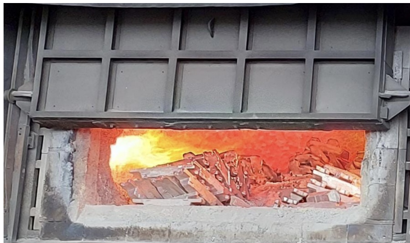
Figure 1. Aluminium smelting furnace, located at Everest Company ltd.
